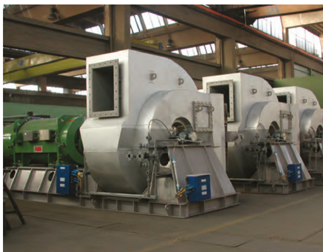
◆ FLUE GAS DELPHURATION
