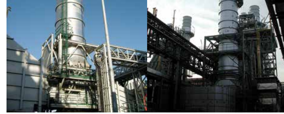
BY PASS SYSTEM - GT GE FR6 BY PASS SYSTEM - GT GE FR6
