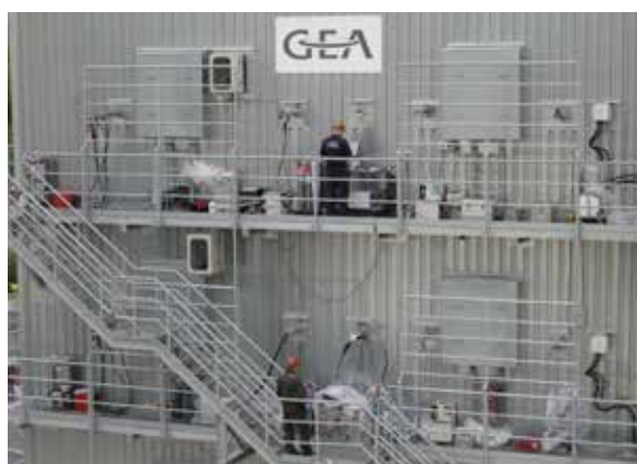
Figure 3. VDZ measurements at different levels of the SCR reactor in the Rohrdorf works.
