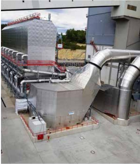
Figure 5. DeCONO x plant in the Allmendingen cement plant.
