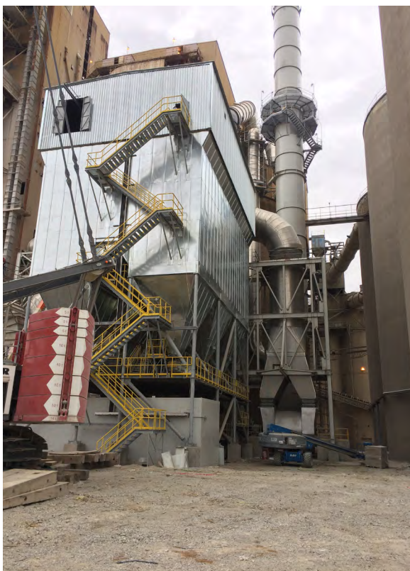
Since commissioning over a year ago, Boldrocchi's 'one lift' baghouse is achieving all expectations.
