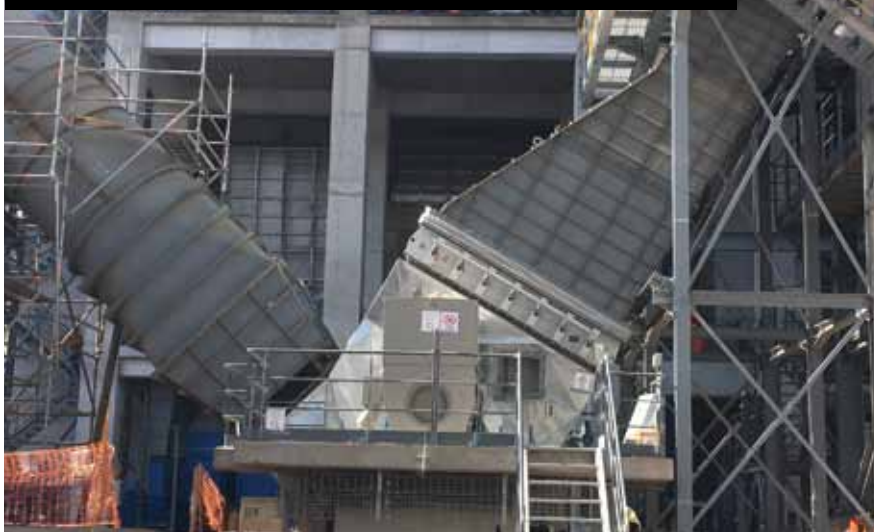
Installing the new equipment at the Tula works of Cementos Fortaleza, Mexico
